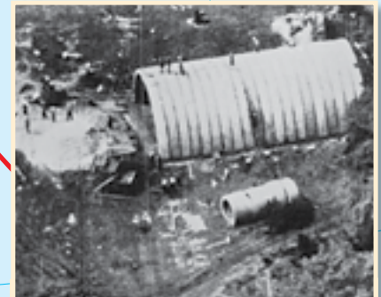
October 23, 1962 A Soviet nuclear warhead bunker is under construction at San Cristobal, Cuba.
